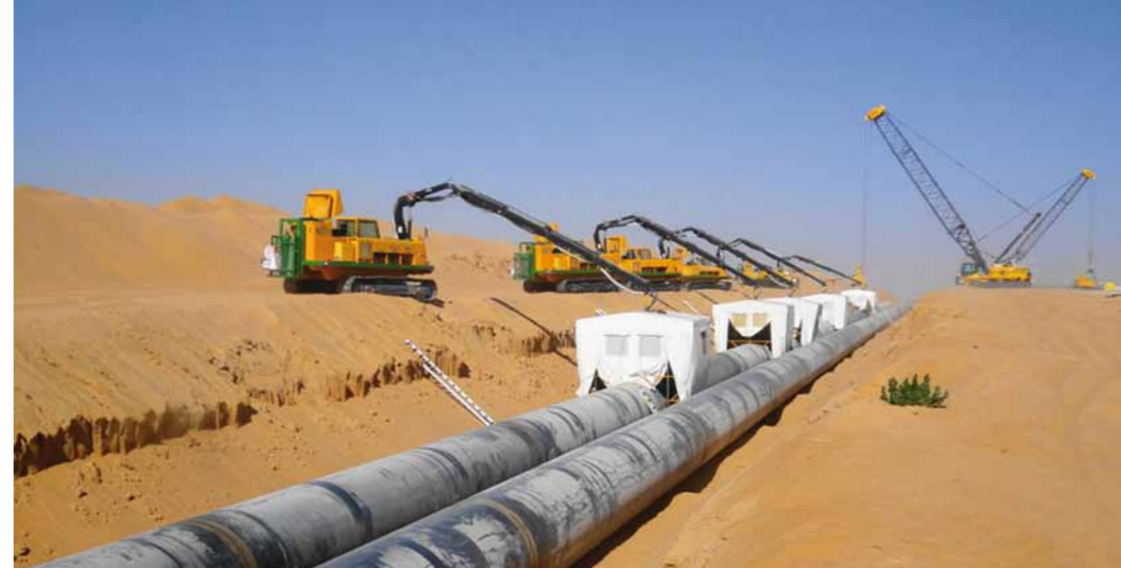
Representative ILF design, major water pipeline, Middle East
