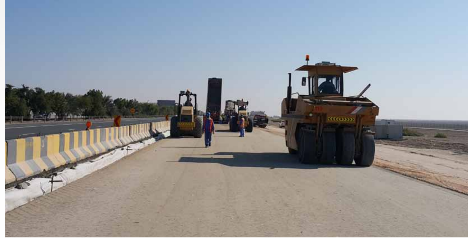
Aggregate base course
